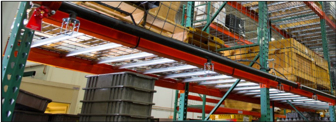
Figure 1. Rack Sprinkler System Installation (Typical)
